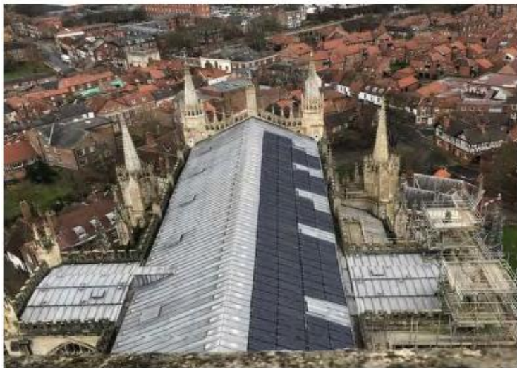
VP 19: From the Top of the Central Tower over the South Quire Roof - Moderate Detrimental
